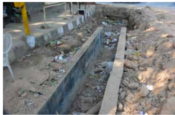
Dry open drains filled with garbage
